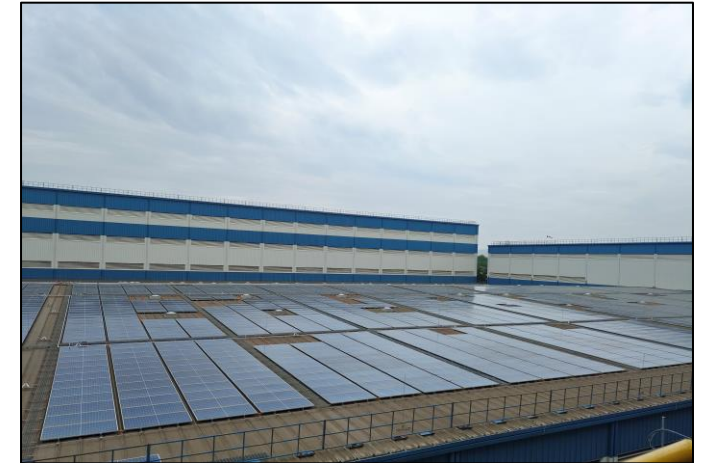
1.264MWp Solar rooftop power plant
